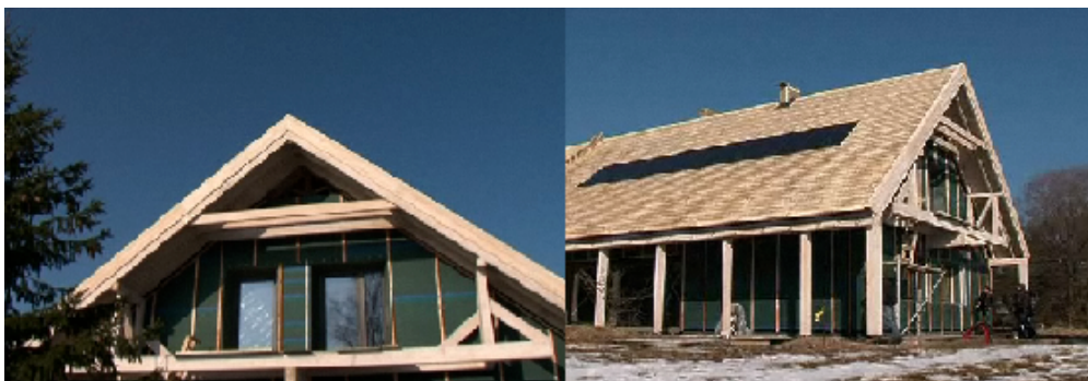
Figure 2.5: The first Passive house in Latvia (in late construction stage) (Ērgle and Baņģieris 2010)
